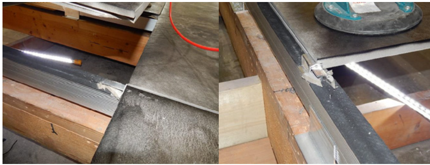
Figure 5. Example of failure mode of the MyDek system.
